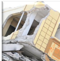
Signs of the earthquake are everywhere.
